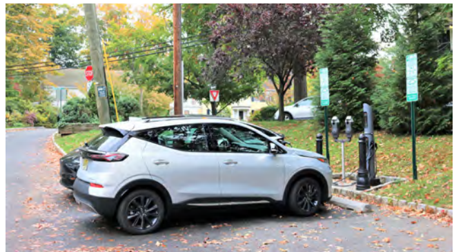
Public Electric Charging Station at The Woodland
